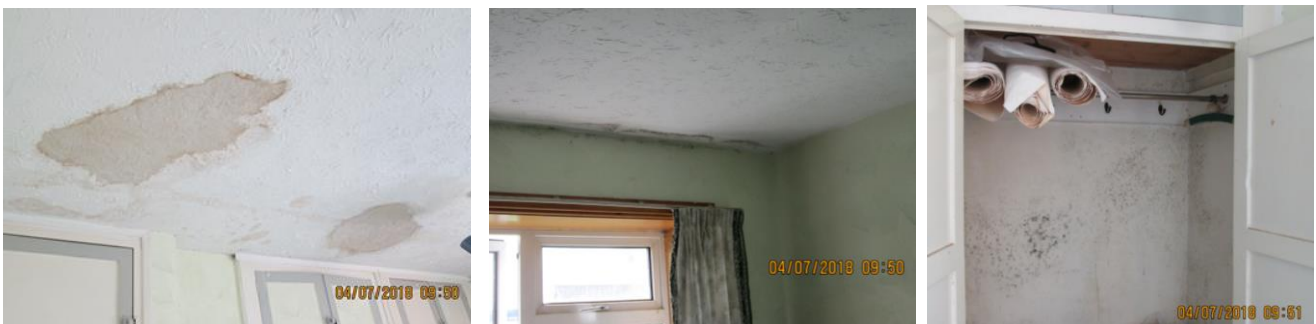
Figure 2.12 Mould issues in property T-01 where a leak (unknown cause) had resulted in mould patches on ceiling near eaves, patches / spots on walls, and damp in backs of fitted wardrobes (against external wall).
