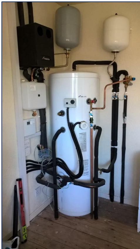
Figure 5.13 hot water cylinder for solar thermal hot water system
