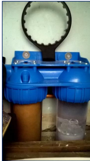
Figure 2.10 filtration system fitted to an InLine hot water system
