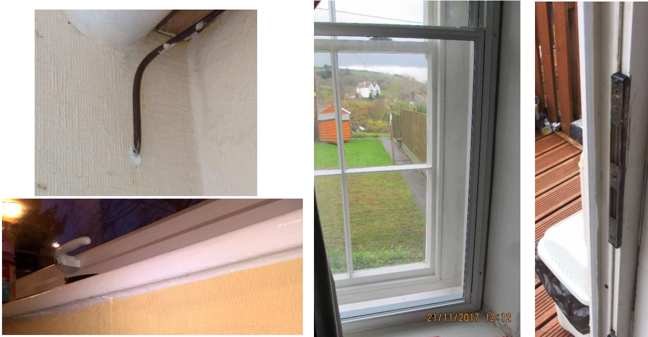
Figure 1.5 – Examples of airtightness measures installed: sealing around pipe inlets, under window-sills, secondary glazing, and EnergySaver window and door sealant
