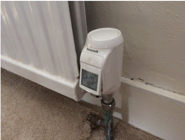
Figure 2.2 Honeywell Smart TRV installed at monitored property
