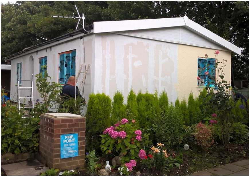
Figure 3.5 Park home retrofit showing joint filler on the InstaClad panels (left) and the final rendered surface (right)
