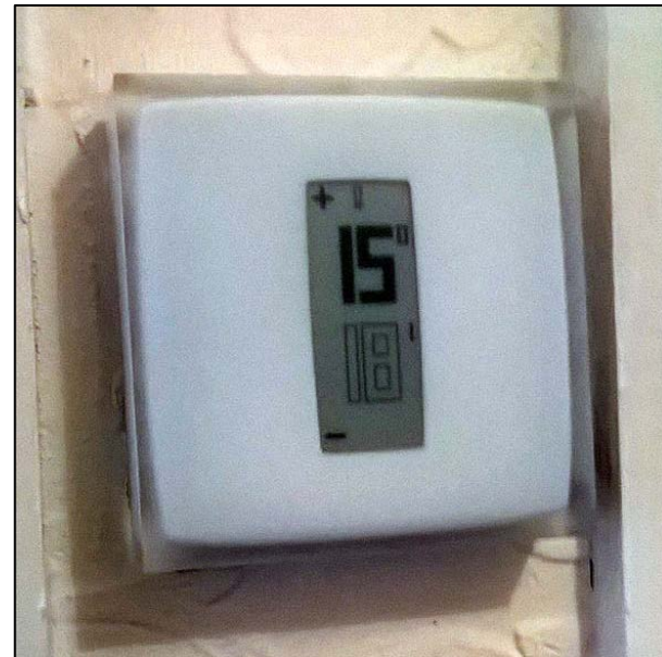
Figure 2.9 Netatmo thermostat in situ
