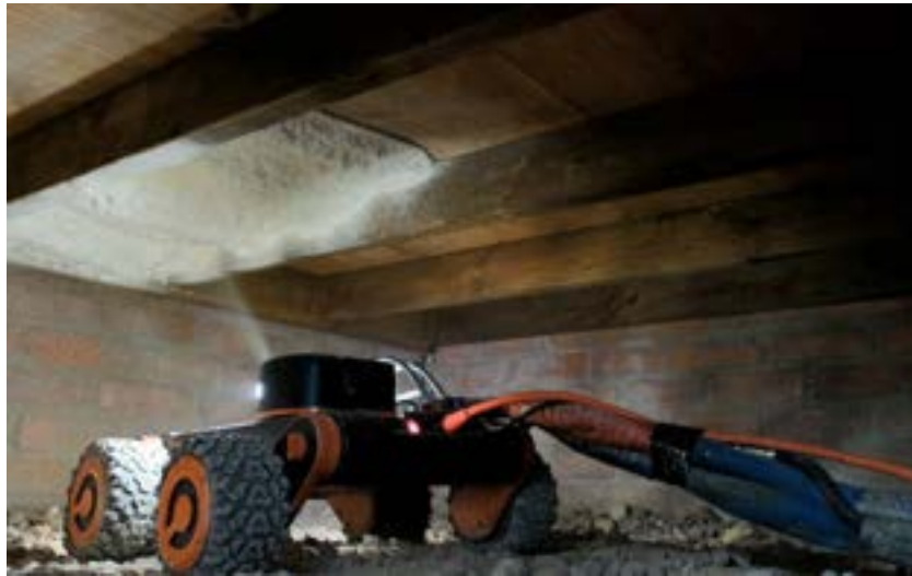
Figure 3.1 (d) Application of insulating spray foam to the under-side of floorboards using the SprayBot
