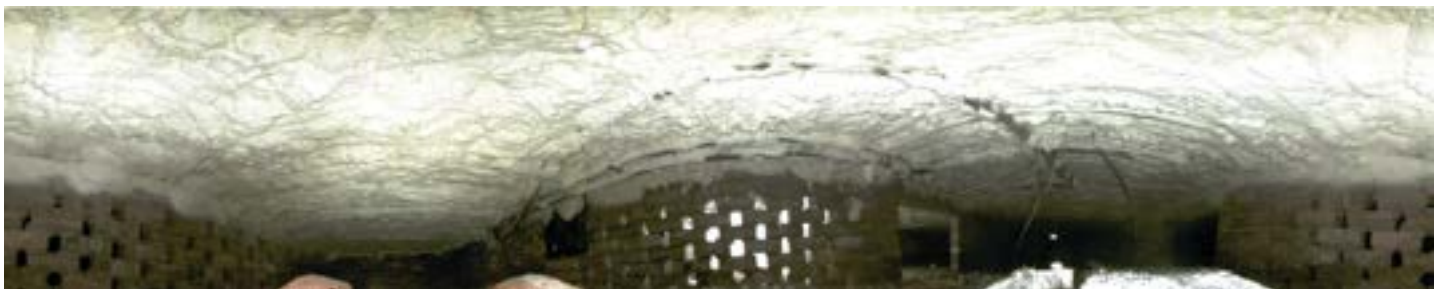
Figure 3.1 (d) Images of the resulting spray foam insulated floorboards from the under-side
