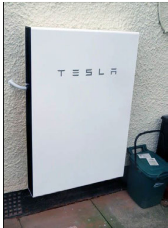
Figure 3.2 External Tesla Powerwall 2 installation
