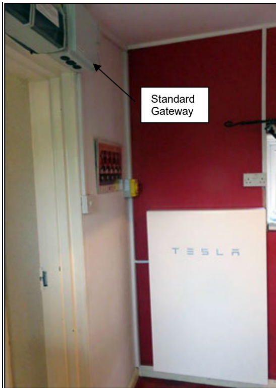
Figure 3.1 Internal Tesla Powerwall 2 installation
