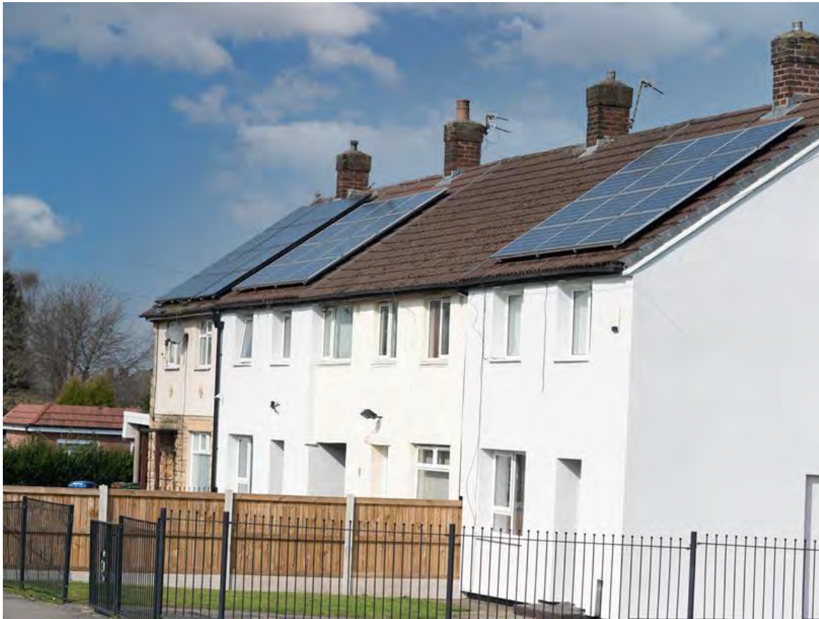
Figure 7.4 Example of Solar PV installation in Stockport
