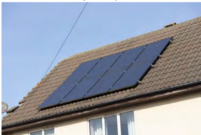
Figure 7.1 Photo of solar PV installations in Sunderland
