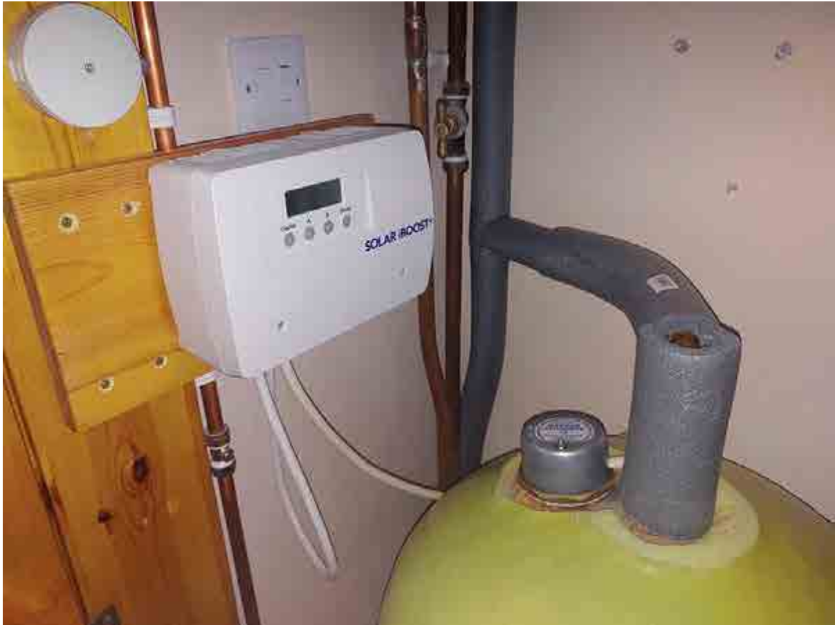
Figure 4.26 Solar iBoost+ solar immersion controller for household W-02 with the hot water cylinder and immersion heater
