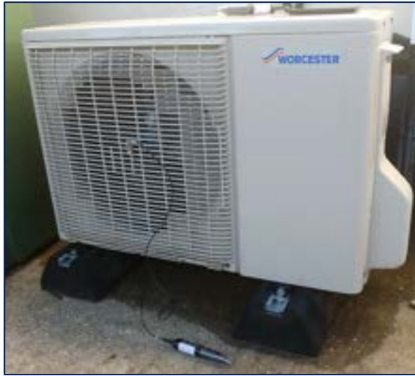
Figure 3.2 Outdoor unit with temperature logger
