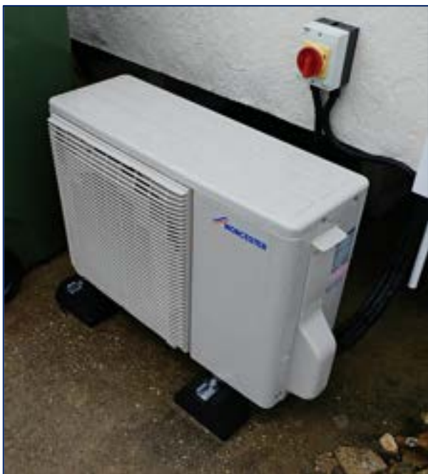
Figure 2.4 Outdoor unit of the ASHP
