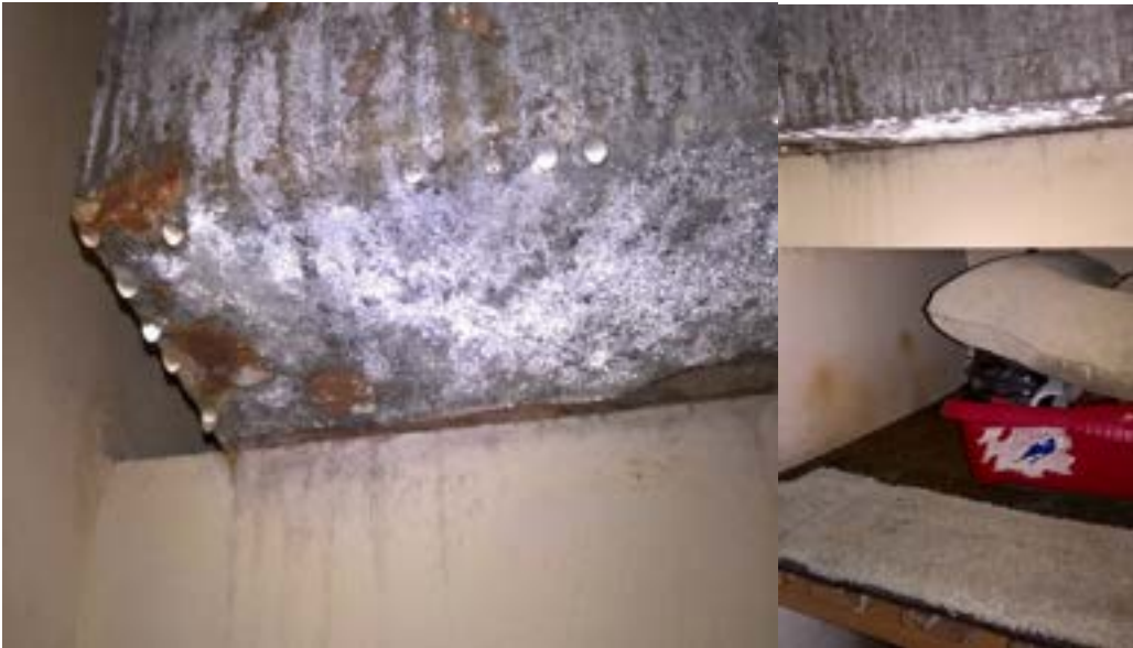
Figure 2.13 Cold water tank causing damp / water ingress.
