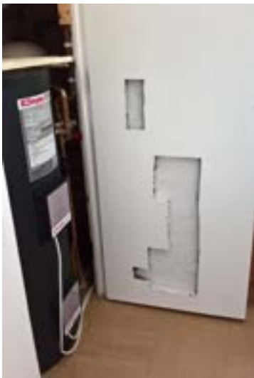
Figure 2.12 (a) example of poor specification of equipment for the space available,
