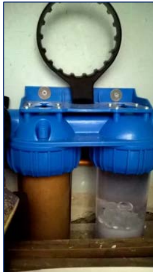
Figure 2.10 filtration system fitted to an InLine hot water system
