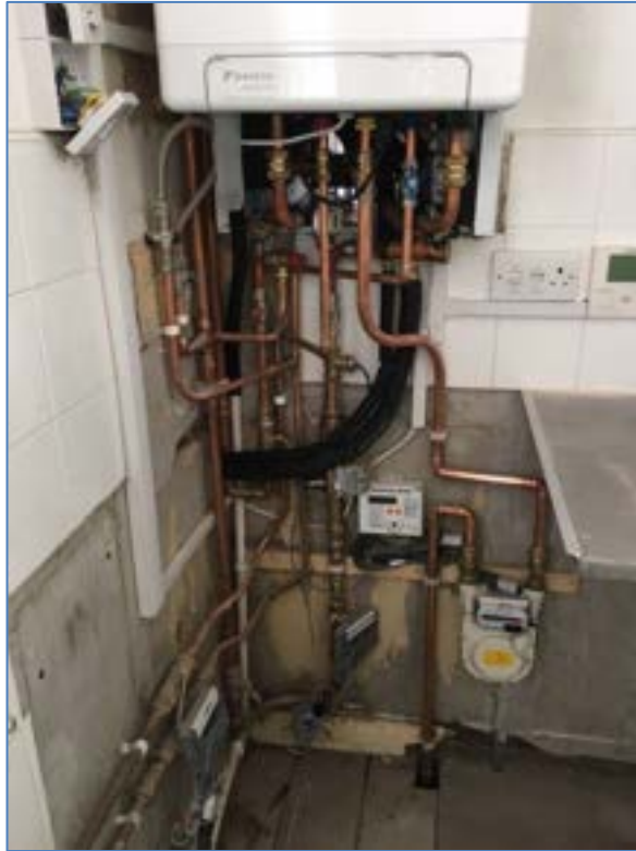
Figure 3.4 heat metering and gas metering installed on the hybrid system pipework
