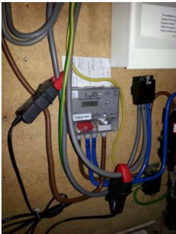
Figure 3.9 showing two current clamps installed on the neutral cable to the heating consumer unit and on the neutral cable to the main consumer unit.
