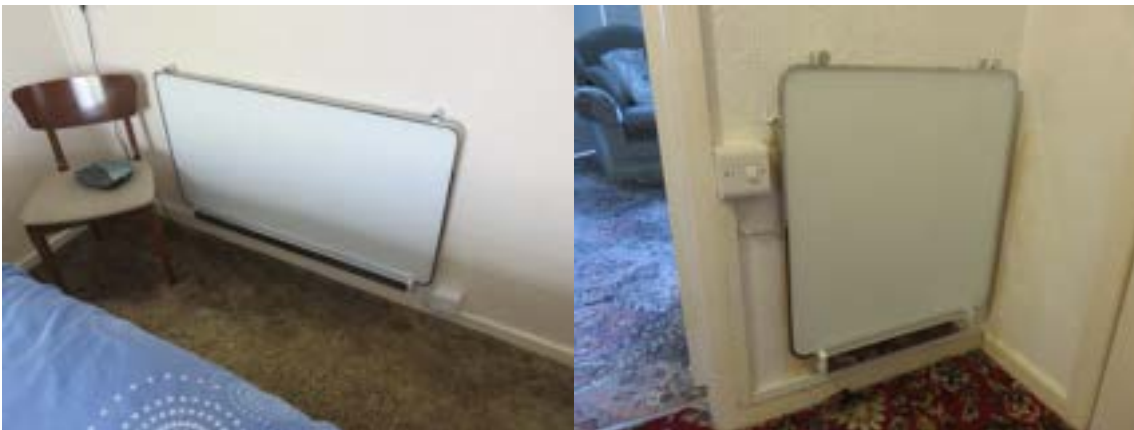
Figure 3.1 Showing GH-518R (left) and GH518B (right) as installed.
