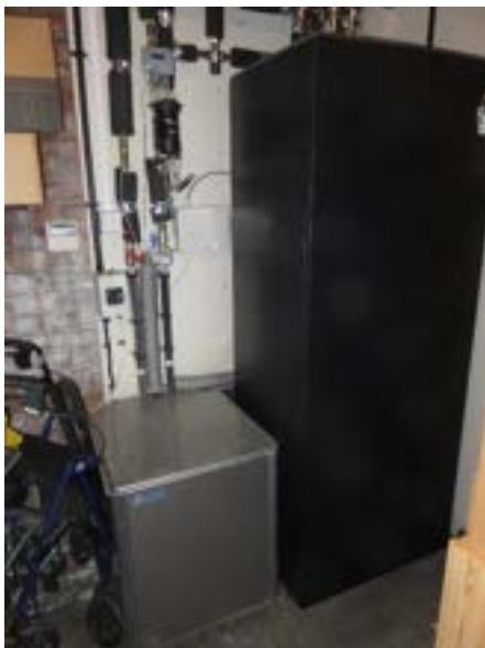
Figure 3.5 Sunamp heat battery and hydrobox
