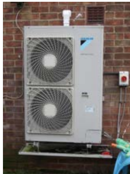
Figure 3.6 Daikin external high temp heat pump unit
