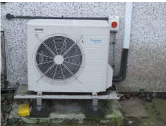
Figure 3.3 external heat pump installed on feet with drip tray
