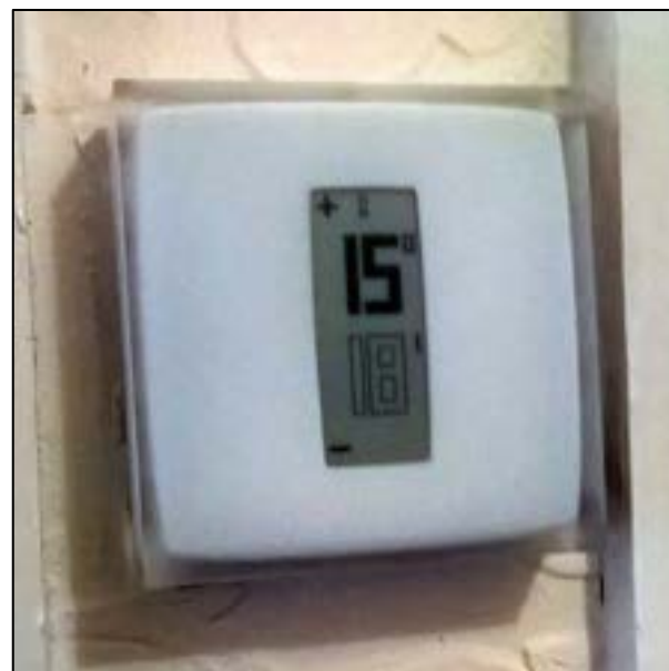
Figure 2.9 Netatmo thermostat in situ
