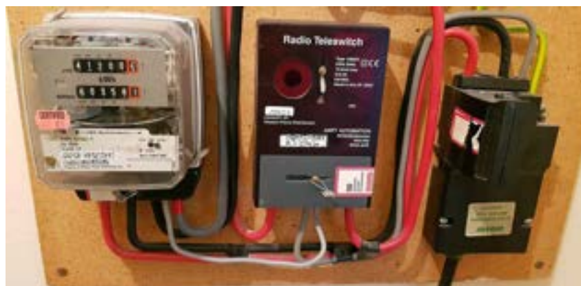
Figure 1.2 Older dual rate mechanical Economy 7 meter with Radio Teleswitch
