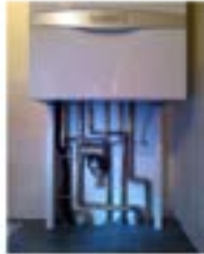
This is a combi boiler. You can see there is no plastic pipework coming from this boiler.
