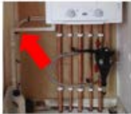
This is a condensing combi boiler. You can easily identify this boiler by the plastic pipework
